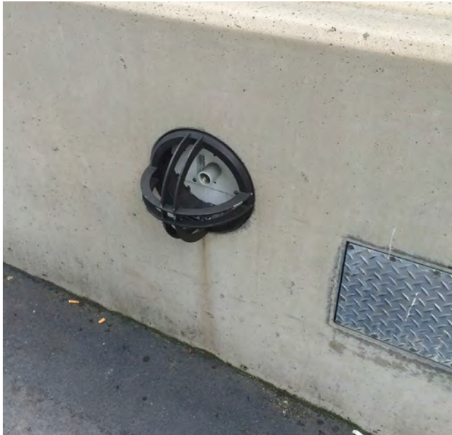
Broken globe light along the Trail on the WMATA wall
