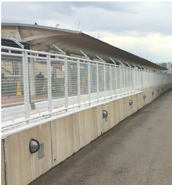
Globe lights along the WMATA wall
