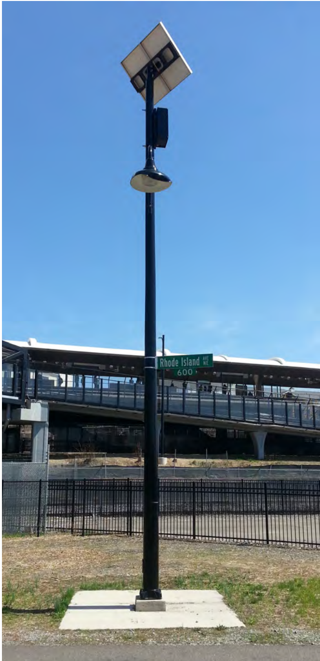
Broken solar lamp post along the Trail at Rhode Island Ave
