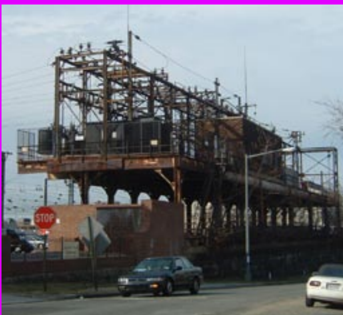
PEPCO substation along Second Street.
