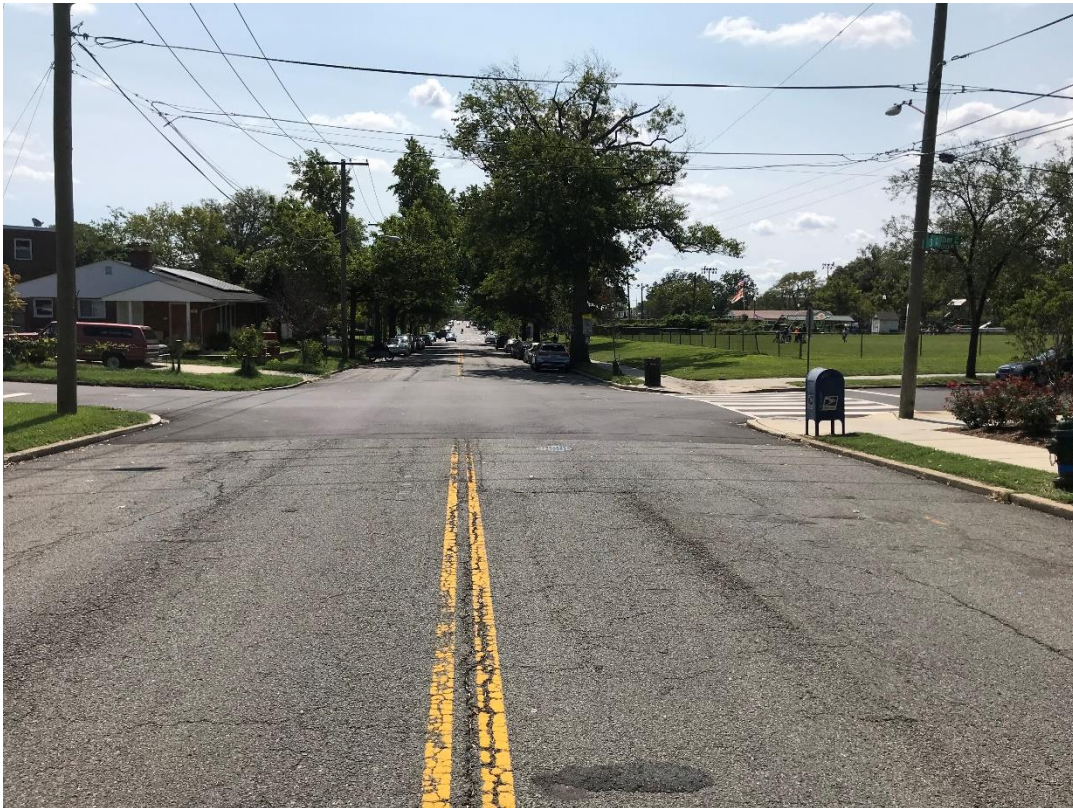
Figure 2: 3 rd Street, NW Northbound Mid-approach
