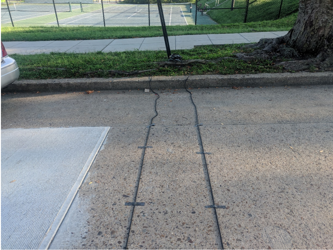
FIGURE 5: Tubes on 300 block of Van Buren Street, NW
