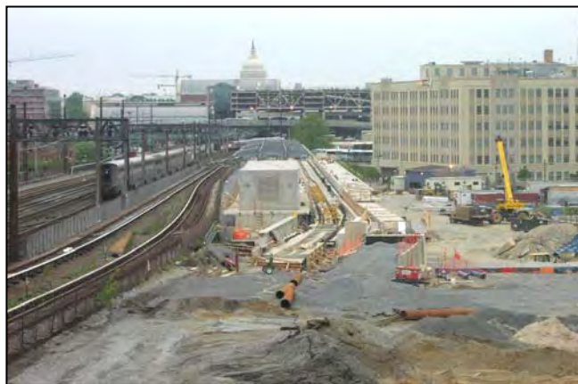
Construction of the New York Avenue Metro Station includes an elevated section of the MBT.
