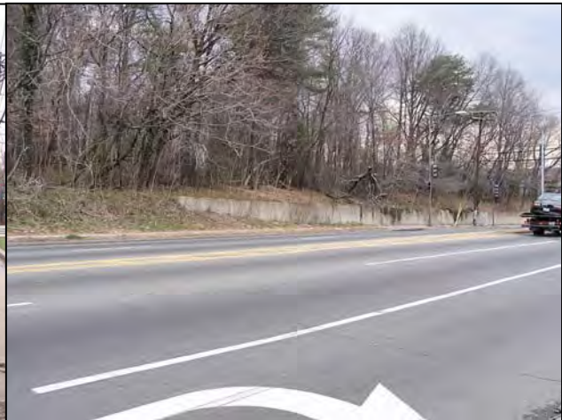
Gap in Riggs Road retaining wall – west of First Place intersection
