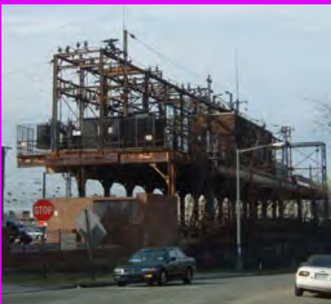
PEPCO substation along Second Street.
